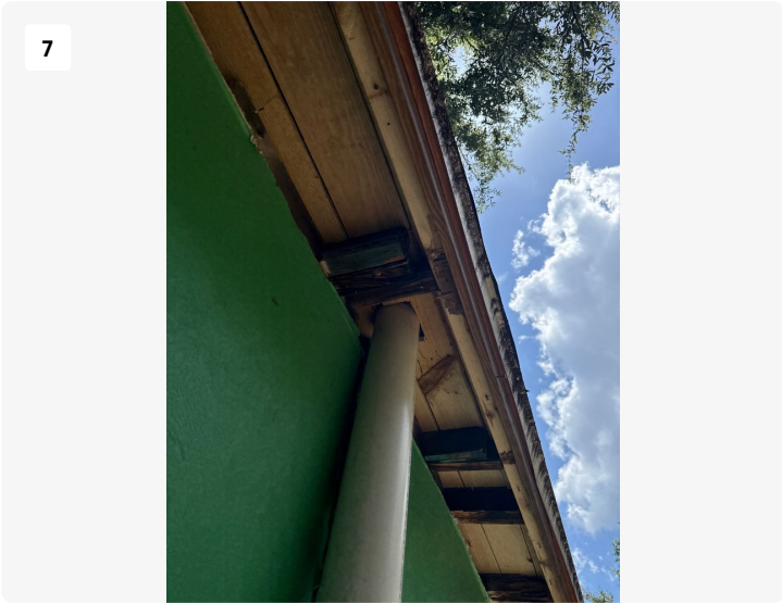
2x Wood rotted.
