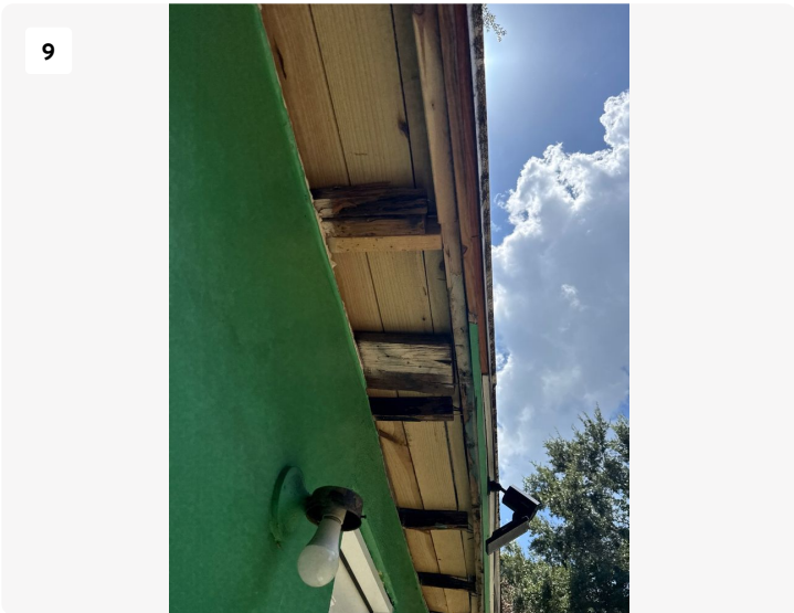
2x Wood rotted.
