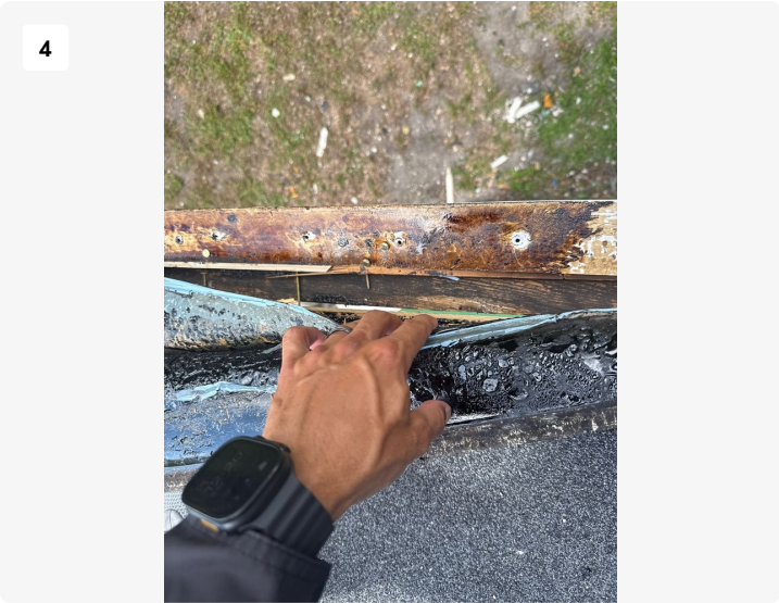
Fascia and drip not properly attached to structure.
