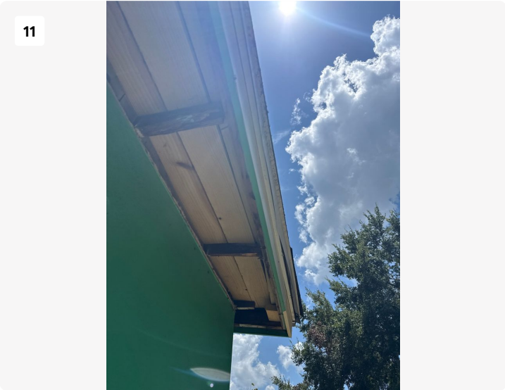
2x Wood rotted.
