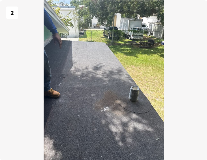
Affected roof area.
