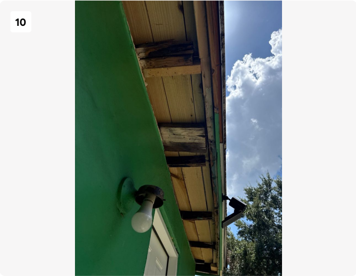
2x Wood rotted.
