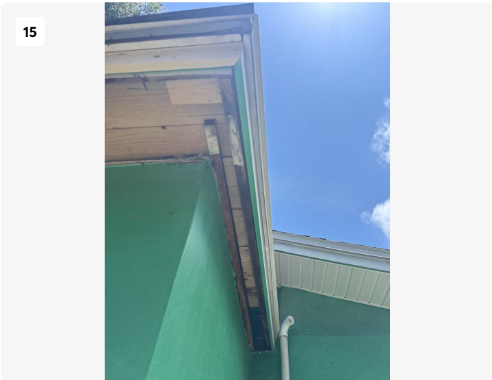
2x Wood rotted.
