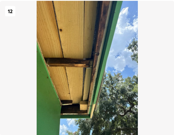
2x Wood rotted.
