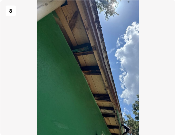
2x Wood rotted.
