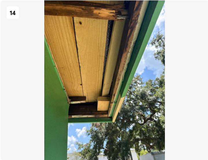
2x Wood rotted.
