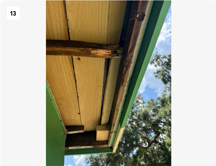
2x Wood rotted.
