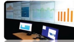
Network Operation Centers
