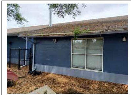
View at rear gutter condition
