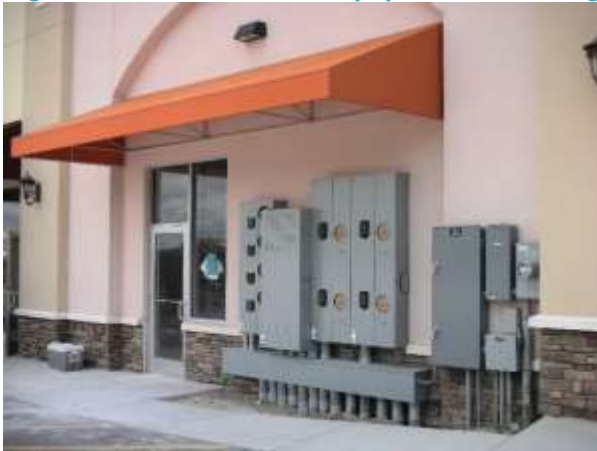
Not Allowed (utilities facing street)
